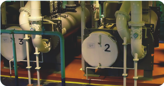
CEMS Engineering built a control system to reduce energy use of industrial air chillers by 30 percent.
